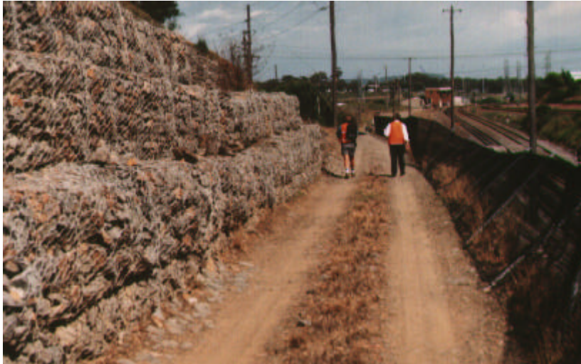
← Section of Main Northern Line corridor constrained by embankment and narrow access road
