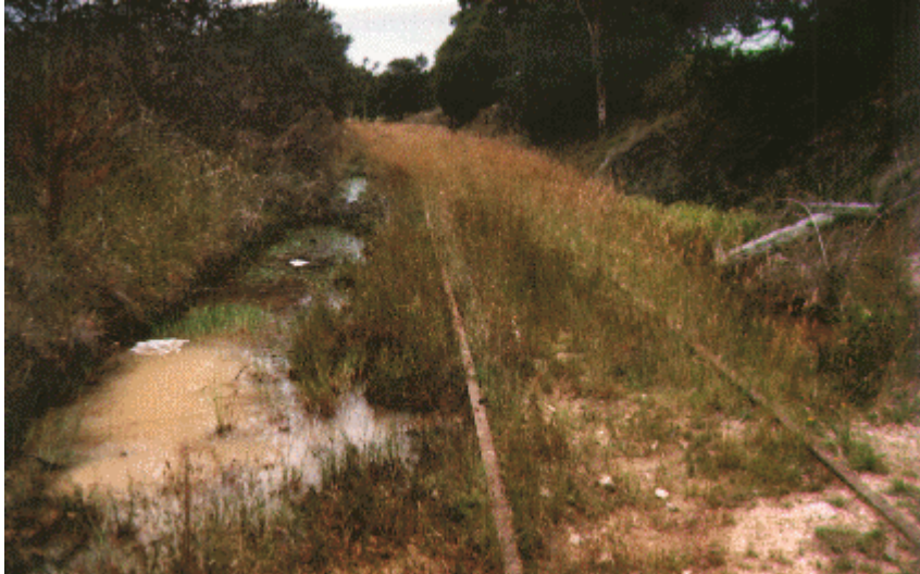
← Section of disused corridor adjacent to F3 freeway, near Braemar showing silt and vegetation build-up over the formation and waterlogged condition.
