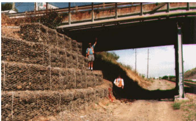
← Maud St Overbridge at Newcastle, showing gabions at abutment and potential cycleway route on a bench above and outside the maintenance access road
